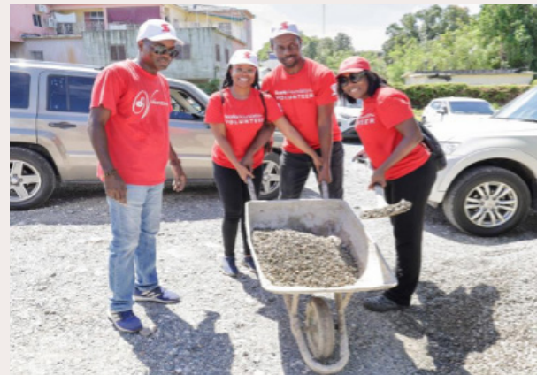
Volunteers help to move gravel at the Busy Bee Early Childhood Institute in St Thomas during Scotia Foundation's Labour Day Project.
